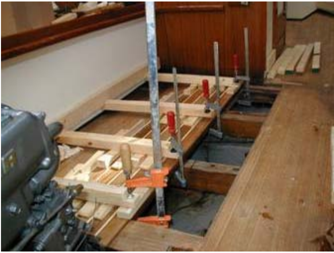
Figure 10 - A system of wedges was designed to hold the planks in place
