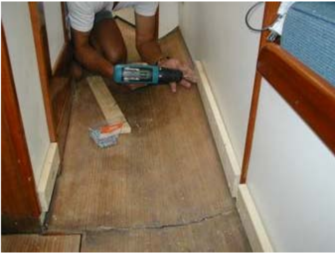
Figure 8 - Furring strips are mounted along the bulkhead to aid in the wedging process
