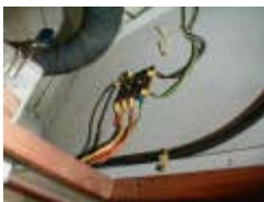
Photo 5 Mast junction wiring detail
