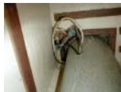
Photo 6 Mast foot wiring close-up
